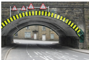
White lines on the road and 'goal posts' on the arch indicating the extent of the signed vehicle height limit
